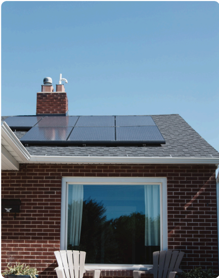
03 · ROOFTOP Rooftop Arrays
